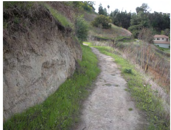
Unstable slope along bench trail.
